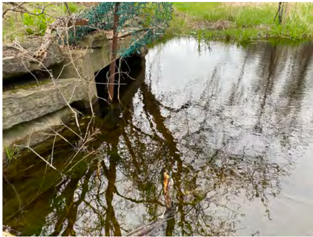
Photo 8: Site WC37; Station AG_10+050 ( Augusta ) - Unnamed Tributary to St. Lawrence; Highway 401 Eastbound, culvert outlet facing northeast
