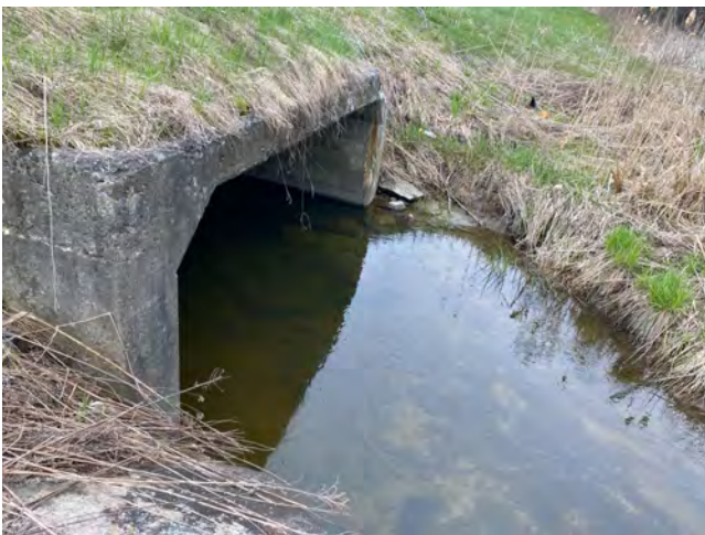
Photo 5: Site WC36; Station ET_24+364 (Elizabethtown) - Butler's Creek; Highway 401 Westbound, culvert inlet facing southwest
