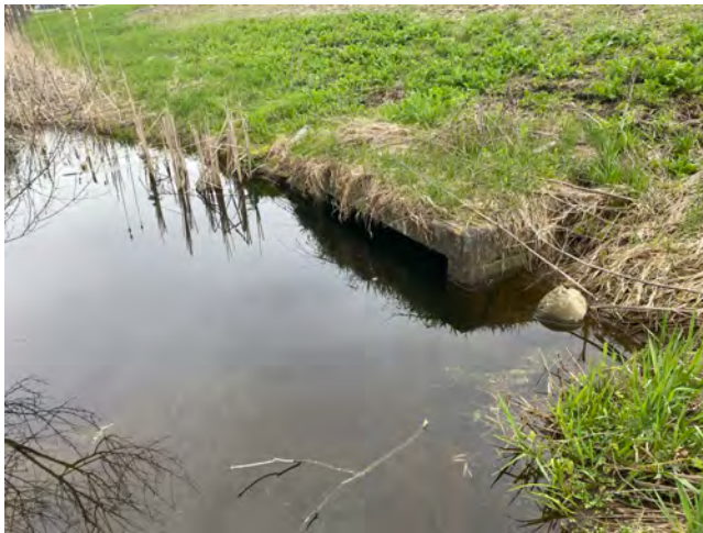
Photo 16: Site WC37; Station AG_10+050 (Augusta) - Unnamed Tributary to St. Lawrence; Highway 401 Westbound, culvert inlet facing southeast
