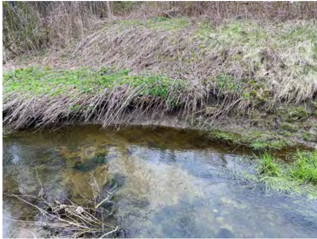
Photo 2: Site WC36; Station ET_24+364 (Elizabethtown) - Butler's Creek; Highway 401 Eastbound, erosion on west bank facing west
