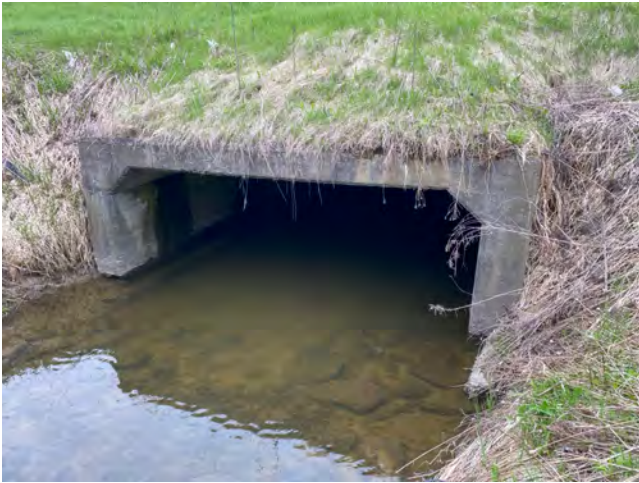
Photo 1: Site WC36; Station ET_24+364 (Elizabethtown) - Butler's Creek; Highway 401 Eastbound, culvert outlet facing north
